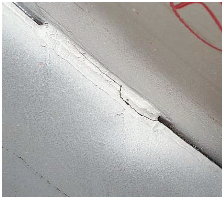
Crack found using magnetic particle inspection.
