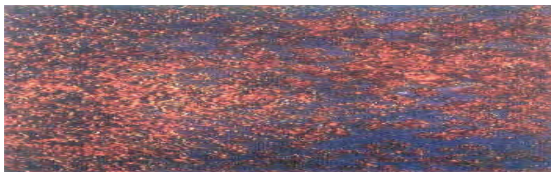
Rust Grade B: Steel surface, which has begun to rust, and from which mill scale has begun to flake.
